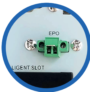
Emergency Power Off (EPO)
